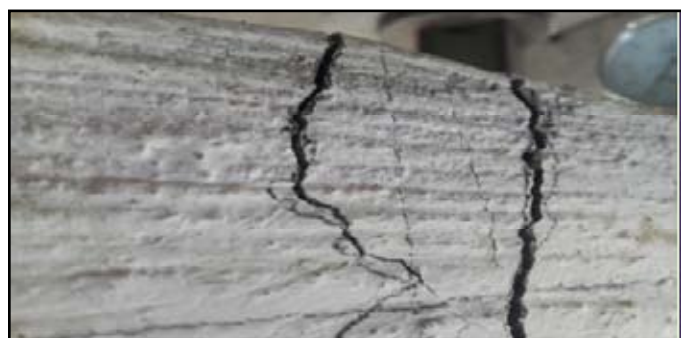
Fig 4: Mode of failure of RC beam
